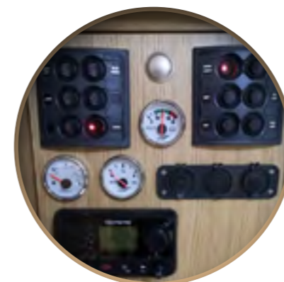
Standard BEP panels with WEMA gauges.
